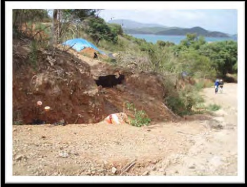
Figure 11: Deep Rill on the side of a dirt road, St. John. (VI RC & D, 2010)
